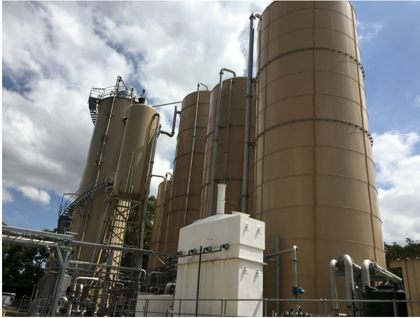
Figure 5.17 Example of an internal circulation (IC) reactor and associated infrastructure installed at a brewery.
