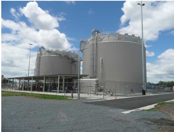
Figure 5.18 Example of two continuous mixed liquor digesters installed at a sewage treatment plant to stabilize waste activated sludge (Gloag et al. , 2014).
