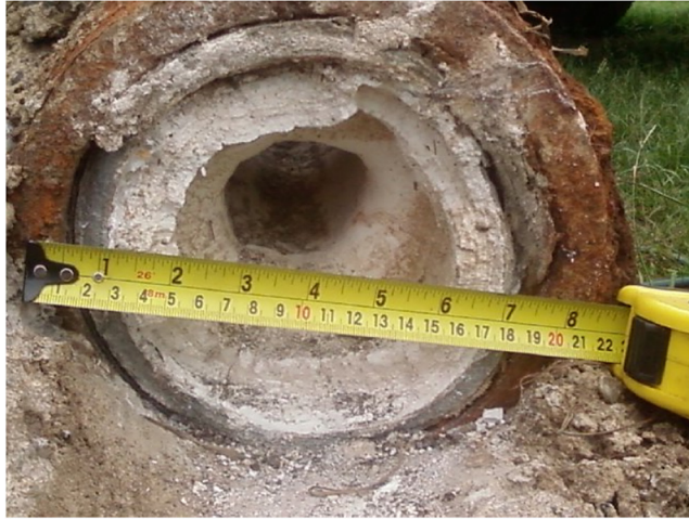
Figure 10.3 Unwanted inorganic scale within water pipework.
