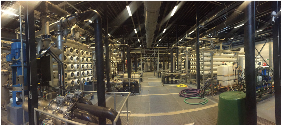
Figure 12.2 (a) Ultra Pure Water Factory Emmen (front) with WWTP Emmen (background); (b) Interior of the UPW Factory Emmen with RO membrane unit in front (photo credits: Arjen van Nieuwenhuijzen, Witteveen+Bos).
