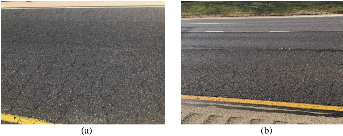
Figure 2-8. Pictures of a) I-90 west to I-39 ramp and b) I-90 MP 17.0
