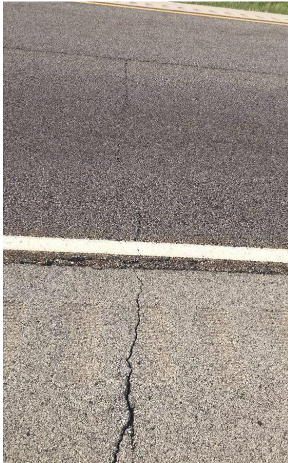
Figure 2-1. Pictures from I-88 at mile post 61 (EB shoulder and mainline)
