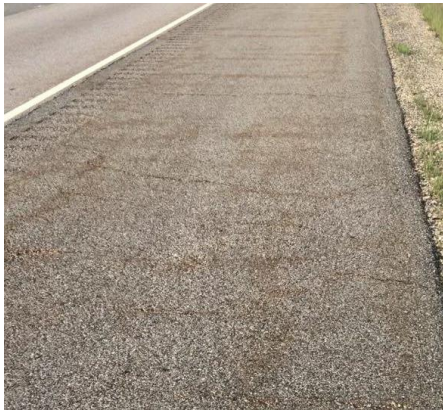
Figure 2-2. Picture from I-88 at mile post 65.9-High ABR rubber modified asphalt (RMA) mix (EB shoulder and mainline)
