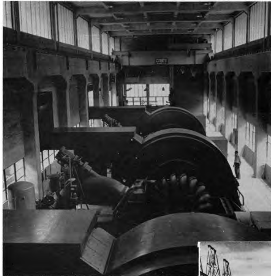
Interior view of Paucartambo's powerhouse situated at Yaupi Bajo, some 11 miles downstream from the Yuncan headworks. The plant houses three generators, each rated 24,000 kva at 0.9 power factor. With the development of a relatively small water storage area, it is possible that a fourth and probably a fifth generating unit may be added to the power plant, increasing its capacity to over 100,000 kva. Three main step-up transformers are installed in a high-voltage switching and transformer station adjoining the powerhouse.
