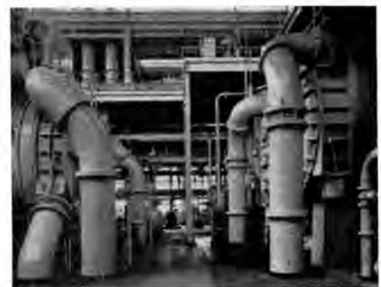
The basement of the turbine hall of Calder Hall A. On the left can be seen the dump condenser used to absorb the steam not required by the turbine. On the right, the conventional condensers of the turbine plant are shown together with the massive one piece concrete base which supports one 23,000 k.w. turbo alternator set.
