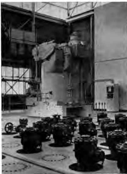
The charging deck of the No. 1 reactor. Some of the control rod actuators can be seen in the foreground.
