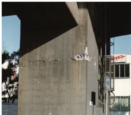
Fig. 11. (Color) Example of horizontal circumferential cracks that occurred in an RC bridge pier. (Image by Keiichiro Sonoda.)
