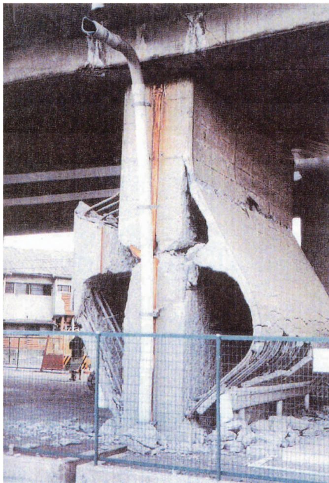
Fig. 1. (Color) Example of the compression failure of an RC bridge pier. (Image by Keiichiro Sonoda.)
