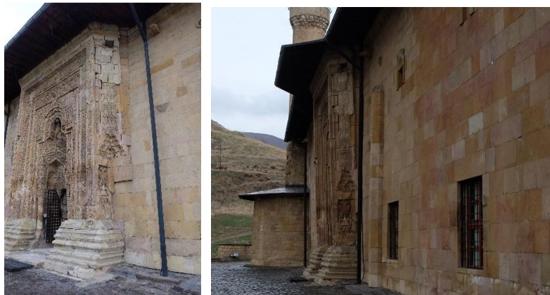
Figure 6: Out-of-plumb deformation of the western façade mosque portal
