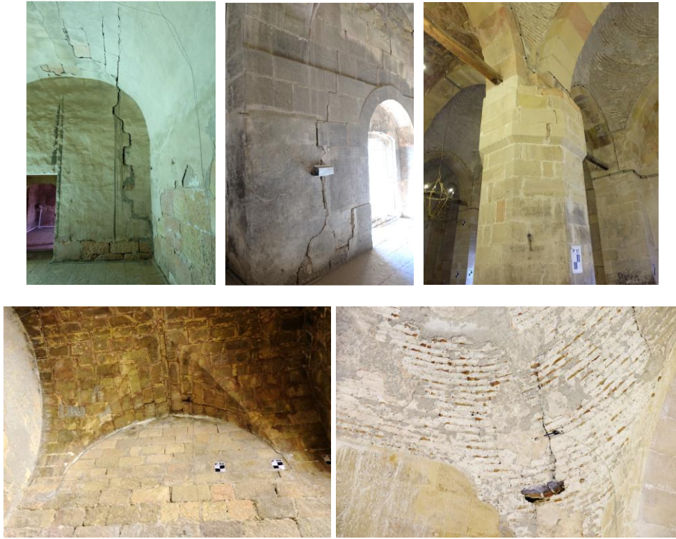
Figure 7: Typical damages on structural members
