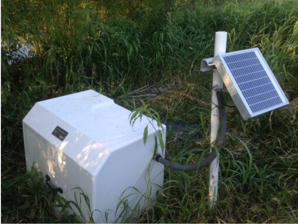
Fig 2. 2 Inflow monitoring equipment at HHN, picture taken August 2019.
