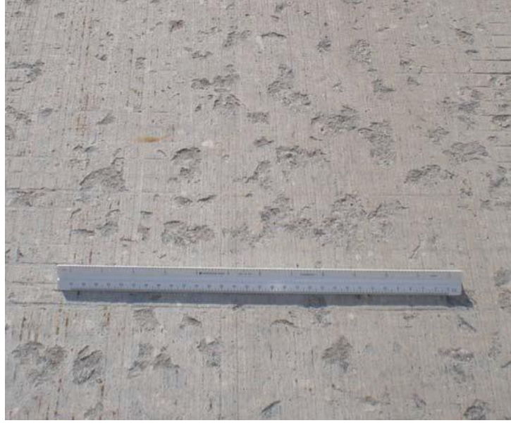
Figure 1.3: Scaling of concrete (Lindquist et al. 2008)
