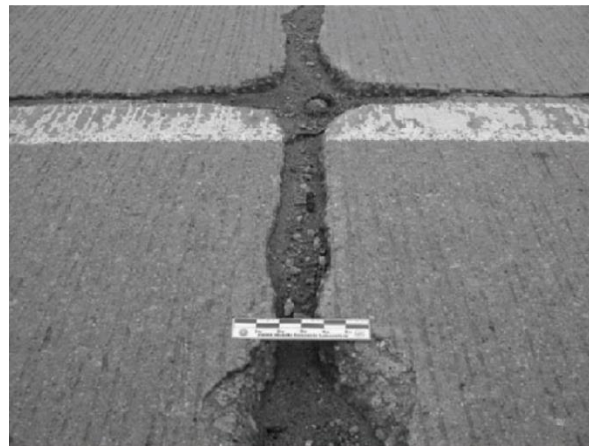
Figure 1.1: Damage at joint (Jones et al. 2013)
