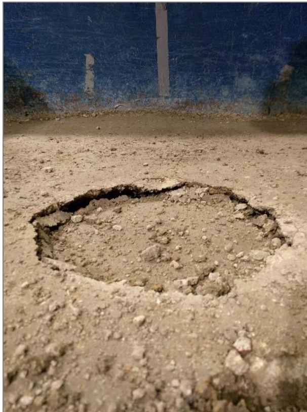
Figure 4.23. Punching Failure at Surface of the VGB Section Due to Cyclic Loading.
