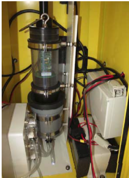
Fig. 6.- Water filling system.
