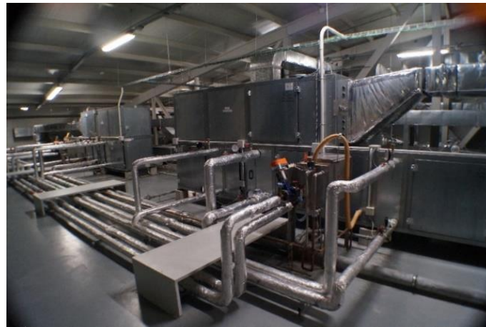
Figure 1. Heating, ventilation and air conditioning (HVAC) system of the surgical suite. In particular, Air Handling Units (AHUs) from OR2 and OR3.
