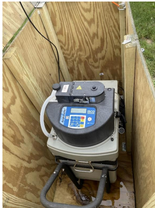
Figure 4. ISCO Avalanche Autosampler at the site
