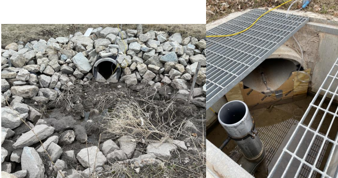
Figure 3. Inlet pipe with weir and forebay shown (left); Outlet structure and outlet pipe with weir (right)
