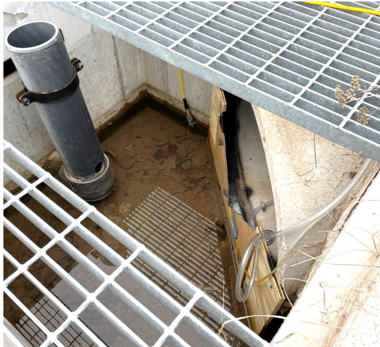
Figure 2. An image of the vertical pipe in the outlet structure and the outlet pipe to the storm sewer
