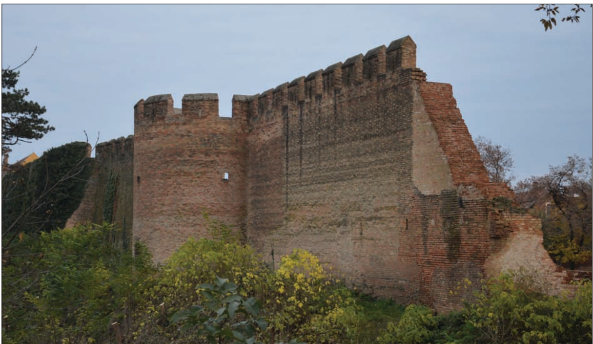
Fig. 28. Crenellated mural tower of the northern wall of Újlak uppertown (The battlement did not preserve its original medieval form.).
