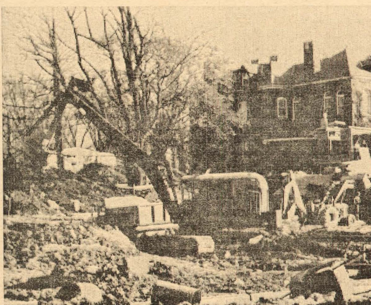
A steam shovel is seen busily working away at what used to be the northern portion of Lower College Road. Contractors are now building the foundation of the new URI half-a-million-book library which happens to be right smack dab in the middle of the street. A pedestrian mall will replace Lower College Road from the intersection of Ranger Road.
