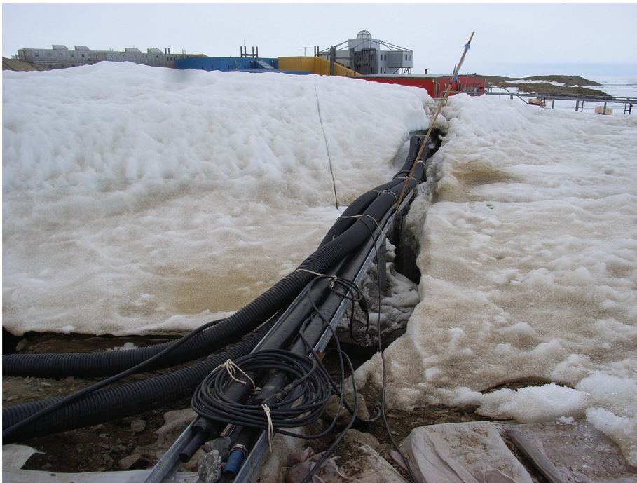
図 21 荒金ダムー屋外水槽の波状プラスチック断熱配管 (第48次隊撮影) Fig. 21. Heat-insulated piping with corrugated plastic material. The pipe runs between Aragane Dam and the outside water tank (photograph by the 48th JARE).
