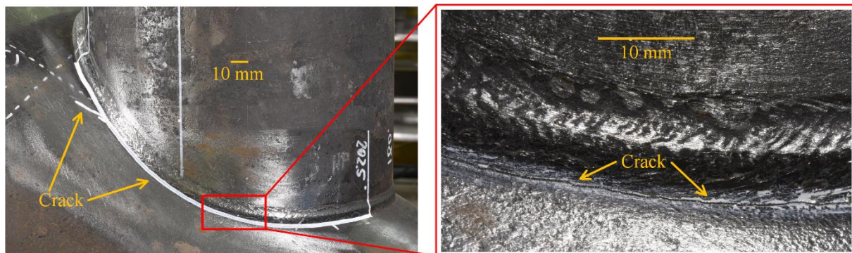
Figure 7. Exemplary crack path after through thickness cracking
