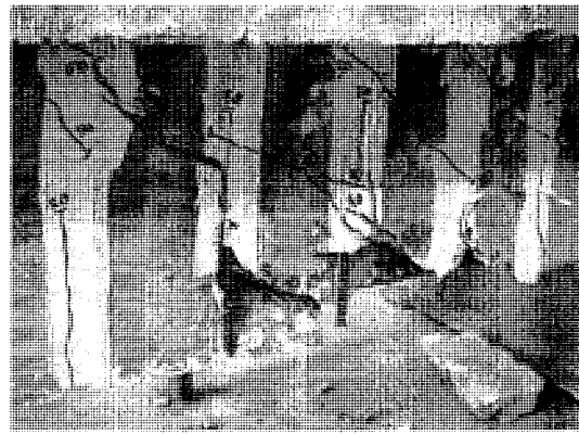
b) Splitting of concrete cover at the longitudinal reinforcement
