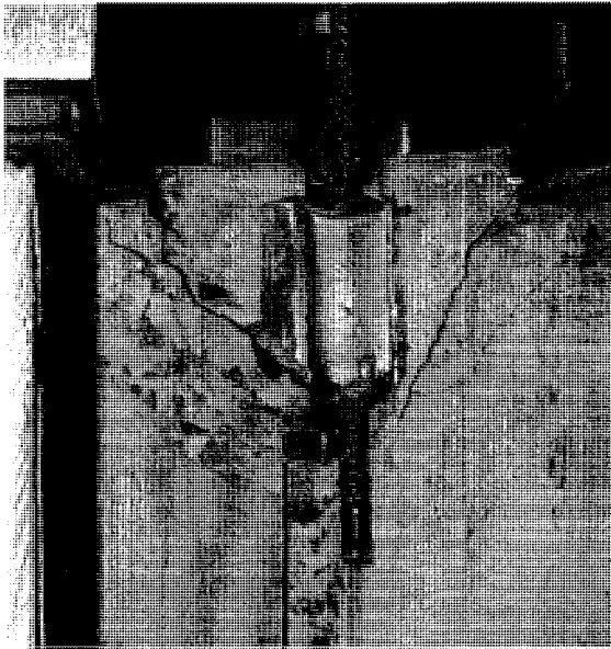
a) Concrete tension failure for C/9.5-E-2.00-6
