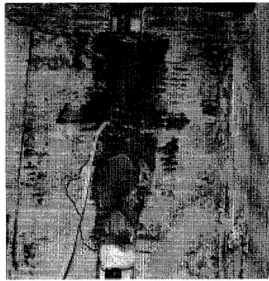
d) Concrete cracking with epoxy cover splitting for C/9.5-E-1.50-18
