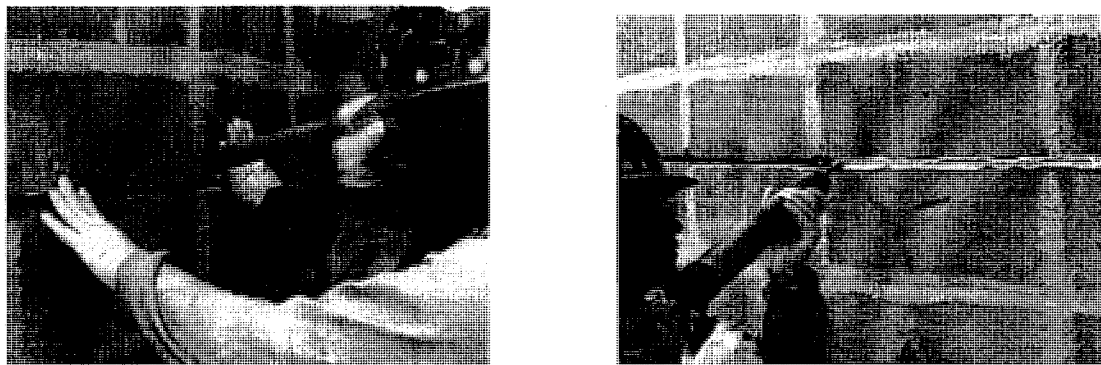
c) putting the FRP rod in the groove. d) additional adhesive is applied to fill the groove
