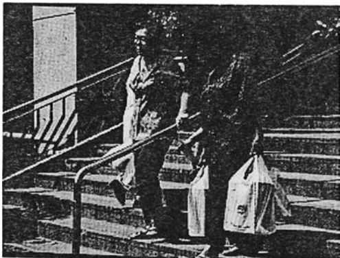
Thai shopping center : Entrance without ramps.
