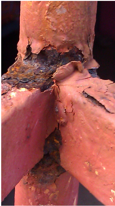
Fig. 3. Failure of coating films can lead to subsequent failure of structures
