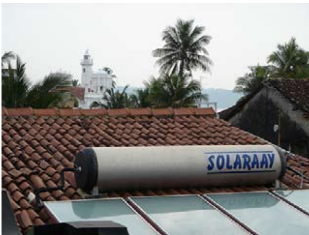
© M. Renner, 2005 Solar thermal panels on the Ocean View Guesthouse. Sri Lanka.
