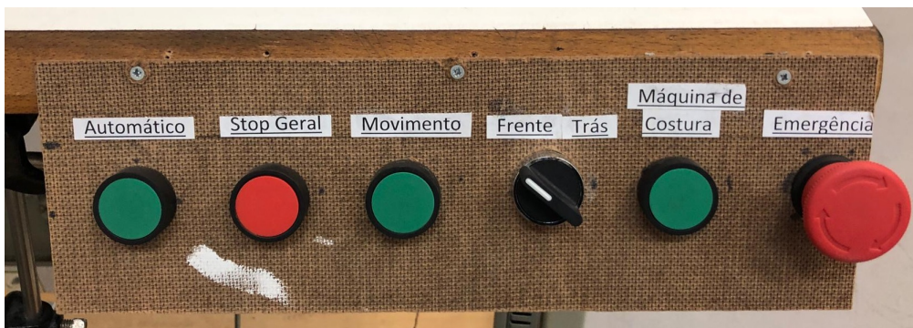
Figure 3.11: Picture of the user's control panel
