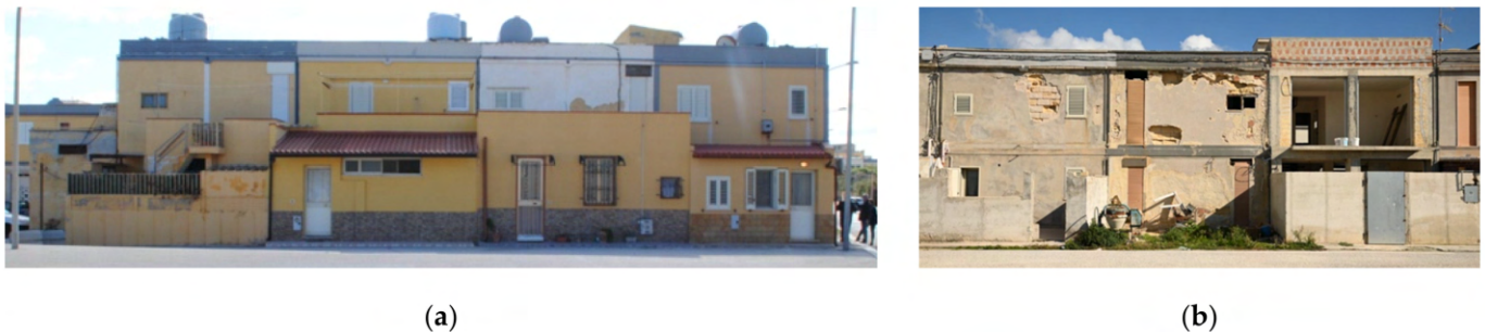
Figure 2. Unauthorized additions in the Cappuccinelli district: private gardens occupied by new rooms (a) and other chaotic modifications (b) in the terraced block named “L”.
