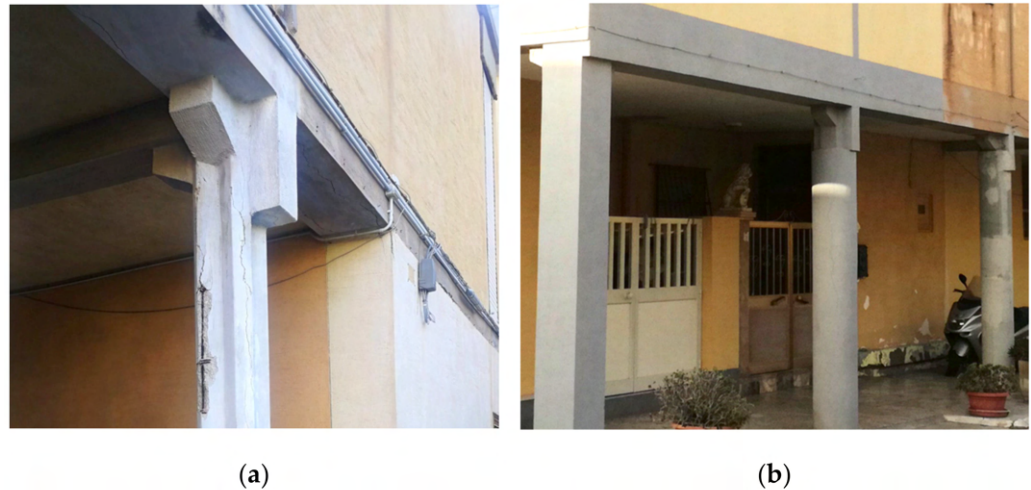
Figure 8. (a) Original shape of pillars designed by Valori. (b) Consolidation of pillars in the portico of court “B”, executed in 2012. Author: Rossella Corrao.
