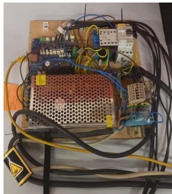
Figure 34: The electronic board for the control of the process.
