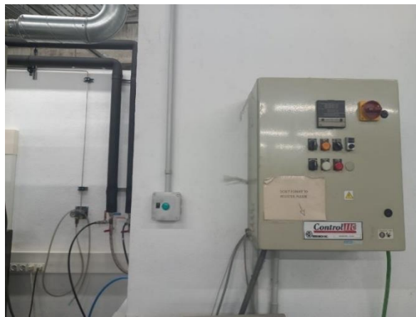
Figure 37: The water-cooling system.
