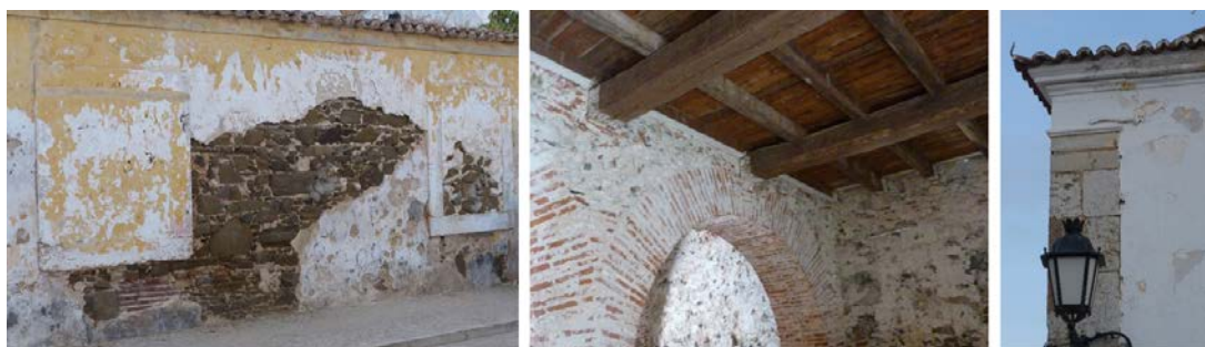
Figure 2: Typical constructive details observed in Vila Real de Santo António: (left) masonry morphology; (middle) diaphragm type; (right) wall-to-wall connections.
