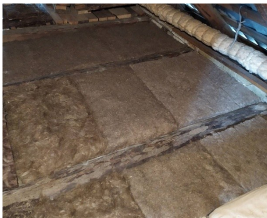
Fig. 1. Thermal insulation slabs made of flax fibers, flax noils, mixture of flax and polyester fibers (from left to right) on the attic flooring
