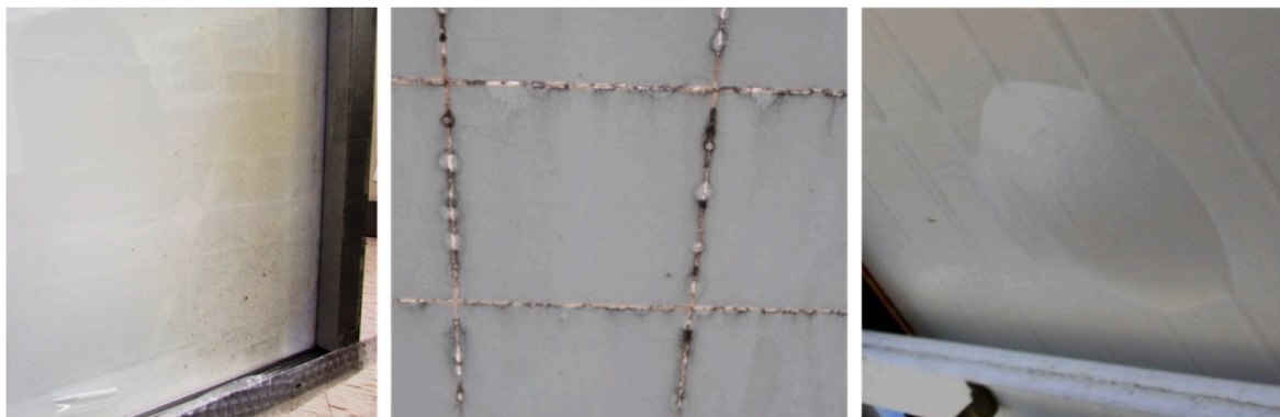
Fig. 6. Examples of backsheet degradation and failure: discolouration (left), cracking (center), and delamination (right). Reproduced with permission from Refs. [25,99].
