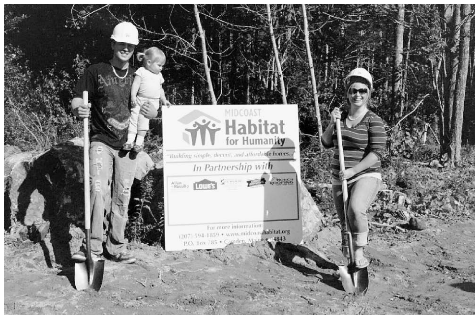
Dan and Amanda Shay and their daughter break ground for their new home in Thomaston.
