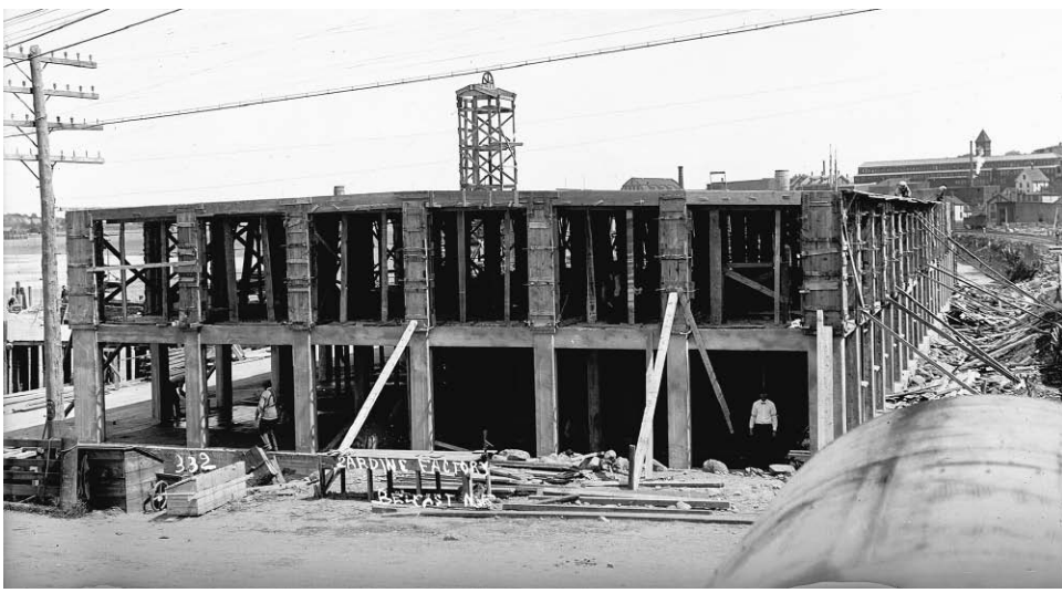
The Stinson Sardine Factory in Belfast being constructed circa 1911. PHOTO FROM THE EASTERN ILLUSTRATING & PUBLISHING COMPANY COLLECTION.
