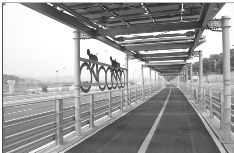
Figure 19. Solar panels covering central bike lane.
