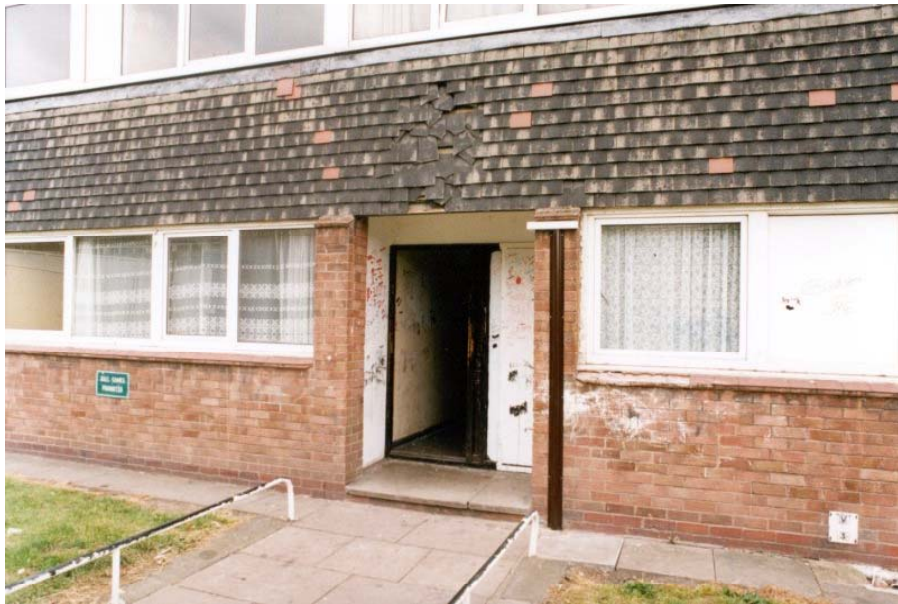
Figure 3. Deterioration of the fabric of a tower block Source: Optima Community Association
