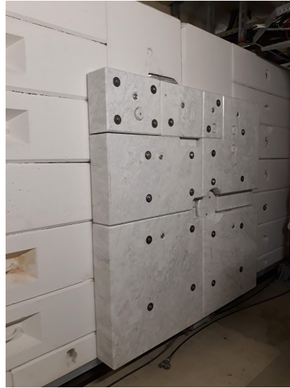
Figure 2.6: The marble shielding on the target shielding wall in the NEAR. In the center the circular hole (closed in the picture) that drives neutrons to the experimental station can be seen.
