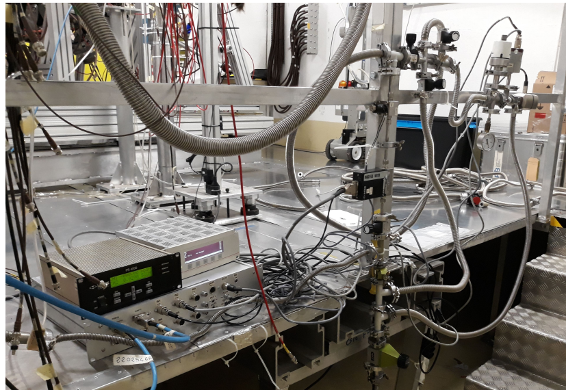
Figure 3.7: The gas regulation circuit for the PPAC in EAR1. In the foreground the Arduino Due device (bottom) with two additional modules to power the sensors. Proceeding to the right, the flow sensor and valve (placed in the vertical direction), the systems of manual valves to connect the circuit to the chamber and the pressure regulation system with the two pressure sensors (above), the mechanical manometer and the Pfeiffer EVR 116 valve. At the bottom, the green valve leads the exhaust gas to the pump.
