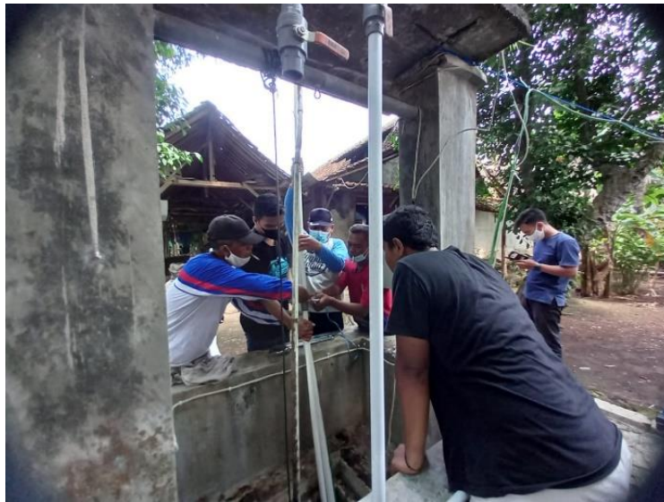
Gambar 3. Upgrade Pompa Air
