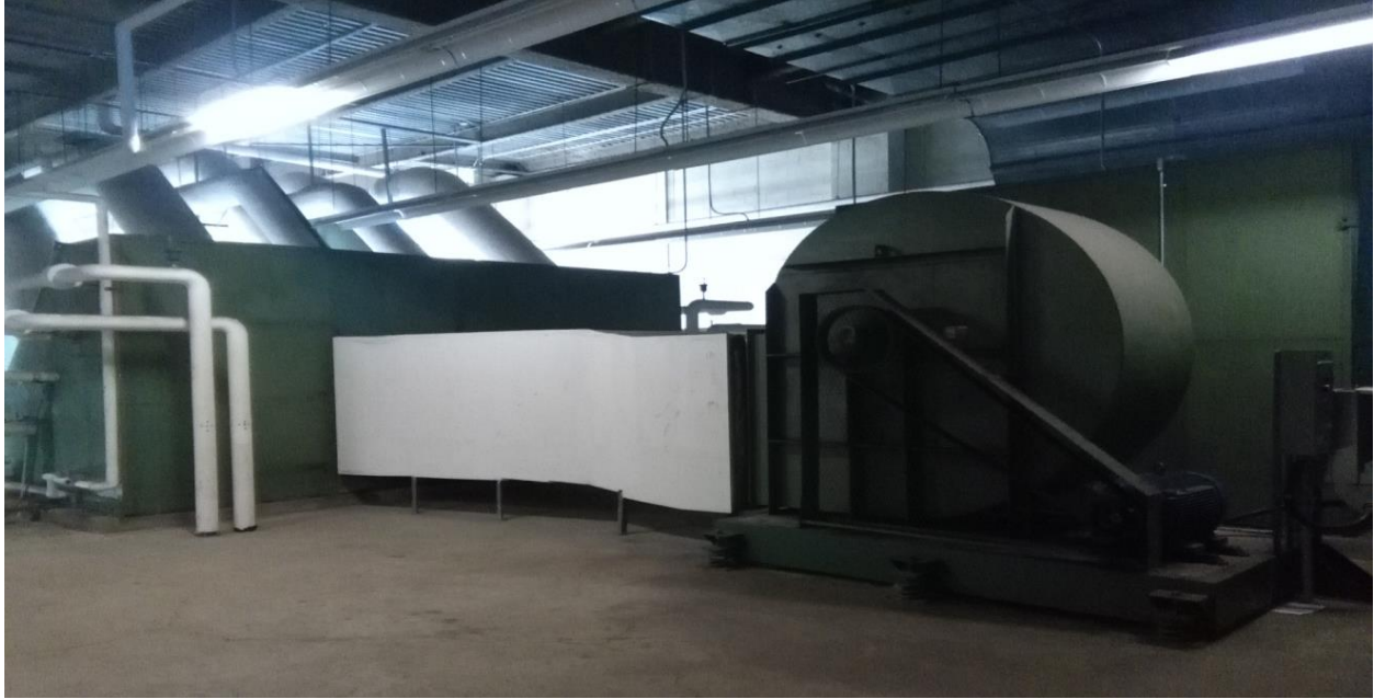
Figure 1.1 Apply fan and the heat exchanger of the AHU 1
