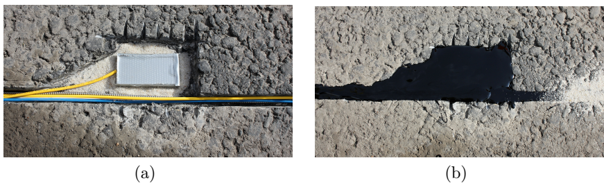
Fig. 3. PDMS-FBG sensor placement in widened milled in groove (a); PDMS-FBG sensor covered with cold asphalt (b).
