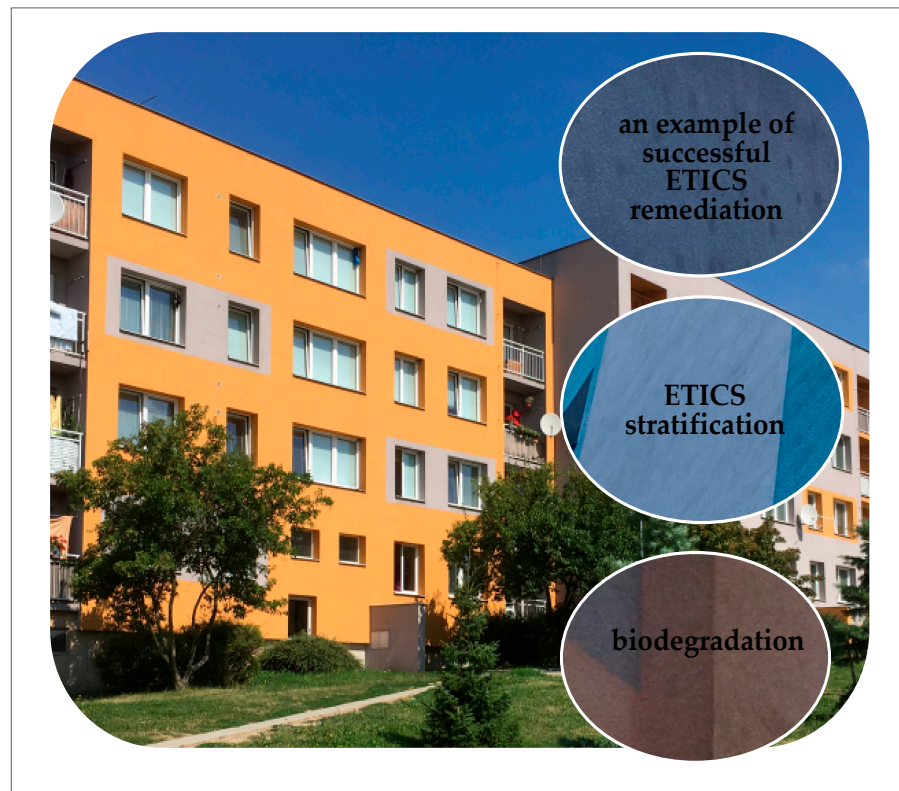
Figure 7. An example of a prefab residential housing after a well-executed ETICS renovation and examples of defects and failures of the external wall due to poor technology in the application of ETICS (photo source: Author's archive [26]).
