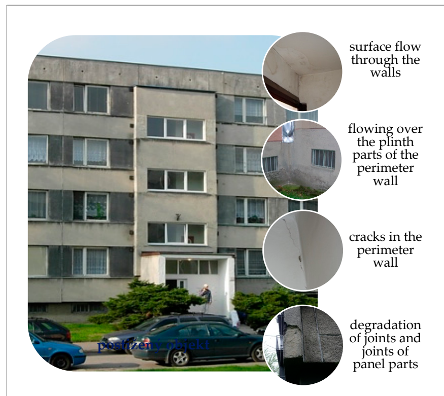
Figure 6. Condition of a prefab residential housing apartment building before the application of ETICS and defects and failures of the external wall (photo source: Author's archive [29,30]).
