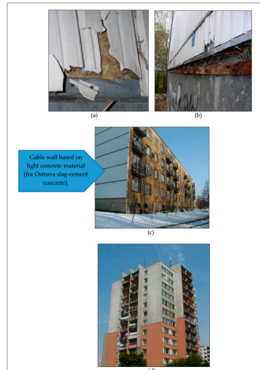
Figure 1. Renovation of prefabricated residential buildings in order to improve the moisture issues of external walls: (a) Degradation of load-bearing strips for anchoring the additional insulation grid and damage to the lamellas; (b) insufficient anchoring of insulating mineral wool; (c) example of post-thermally insulated external wall; (d) example of an additionally thermally insulated building only up to the 6th aboveground floor due to the quality of the material, the use of which at higher floors would not comply with fire safety regulations (Photo source: Author’s archive [29,30]).
