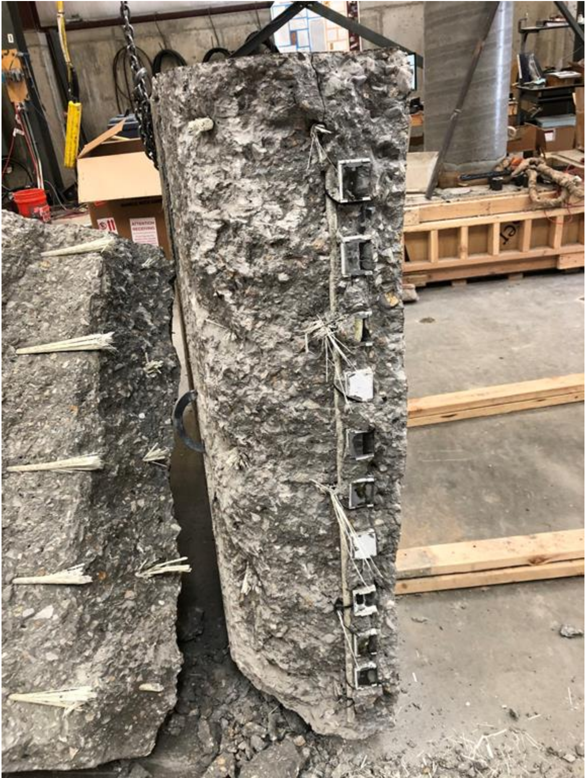
Figure 5-23 GFRP Rupture Exposed
