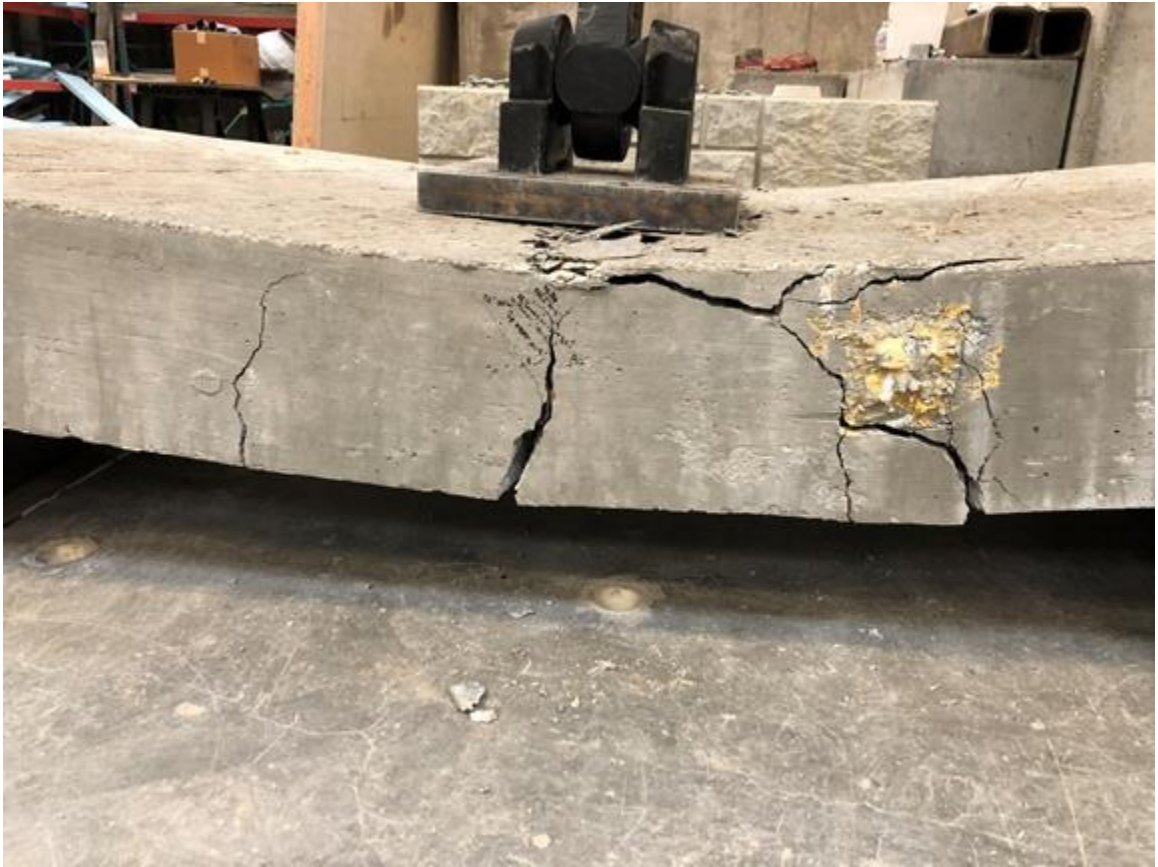
Figure 5-9 Steel Cracking at Midspan
