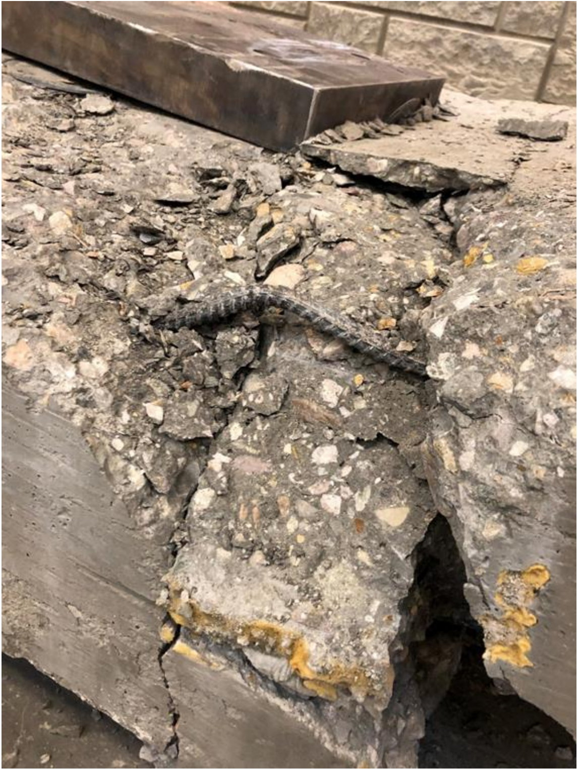
Figure 5-12 Steel Reinforcement Failure
