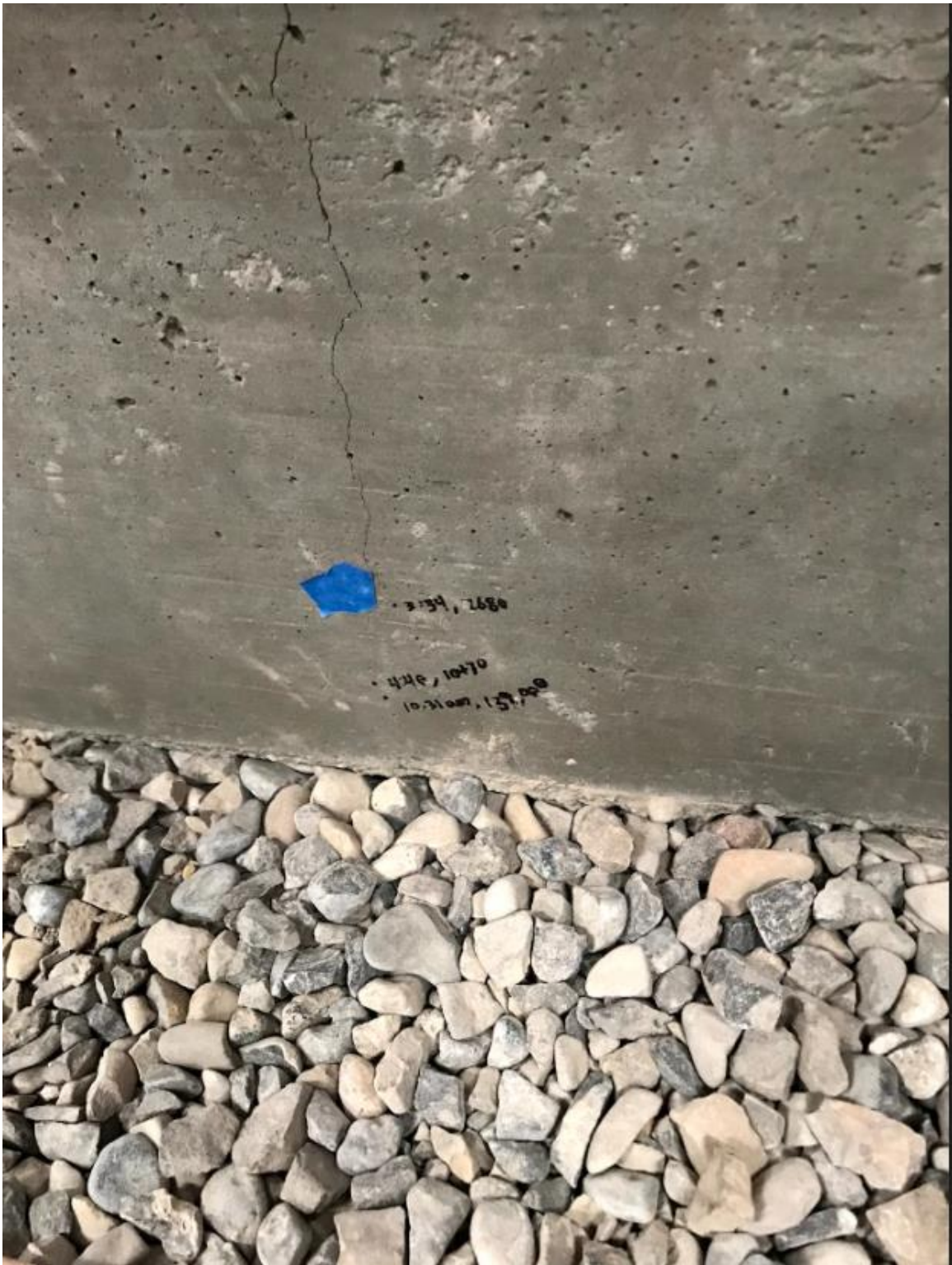
Figure 5-17 GFRP Side Cracking
