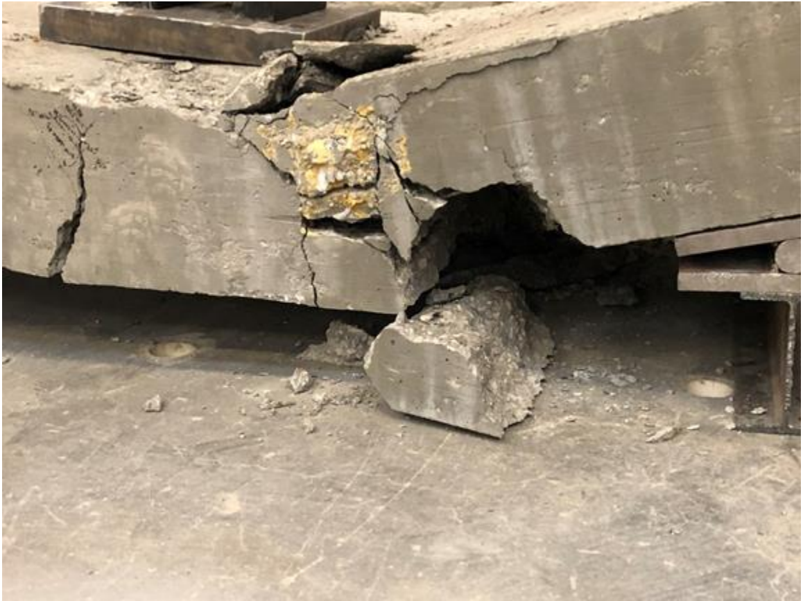
Figure 5-10 Spalling slab with Steel reinforcement
