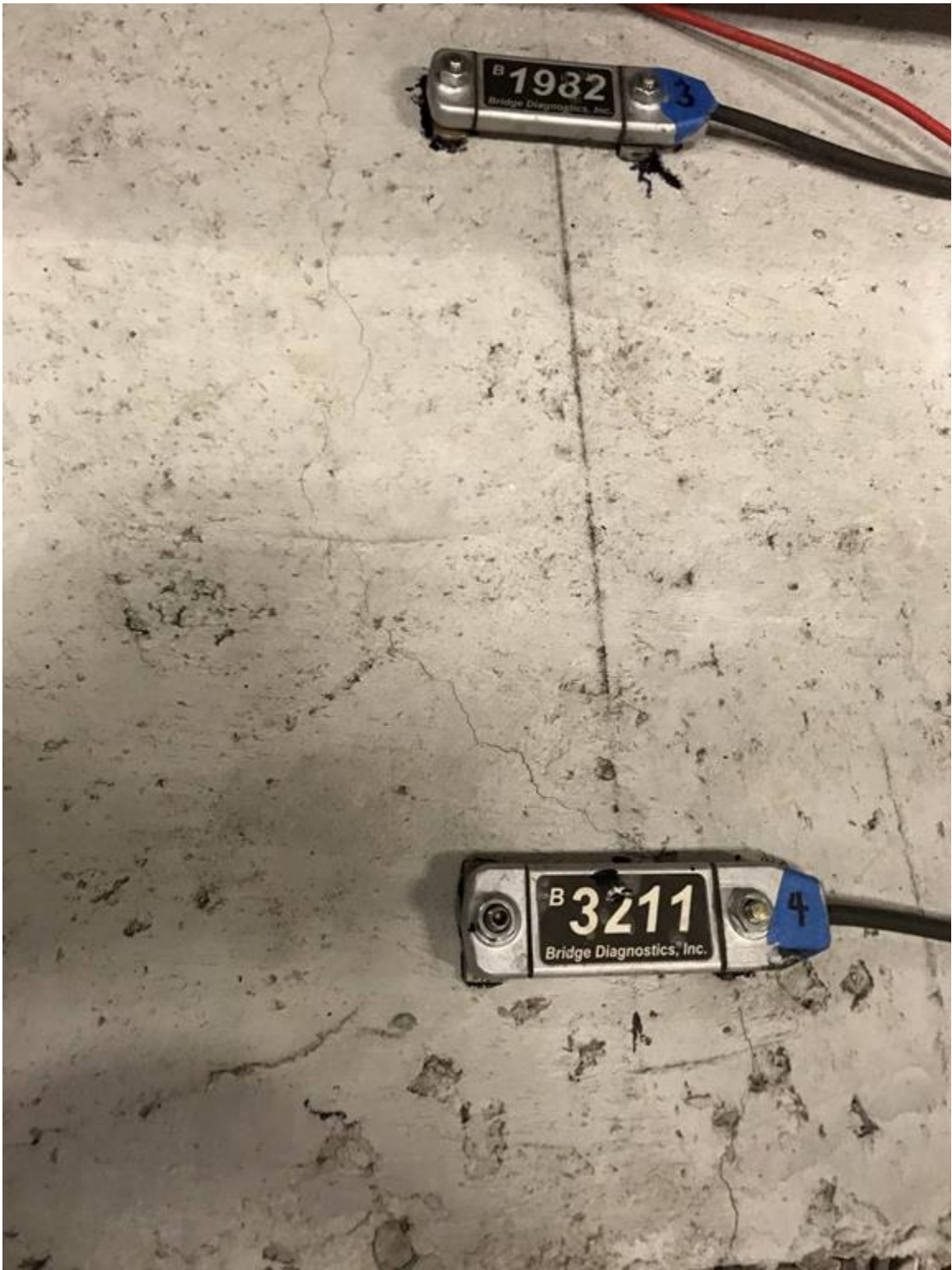
Figure 5-16 GFRP Surface Cracking
