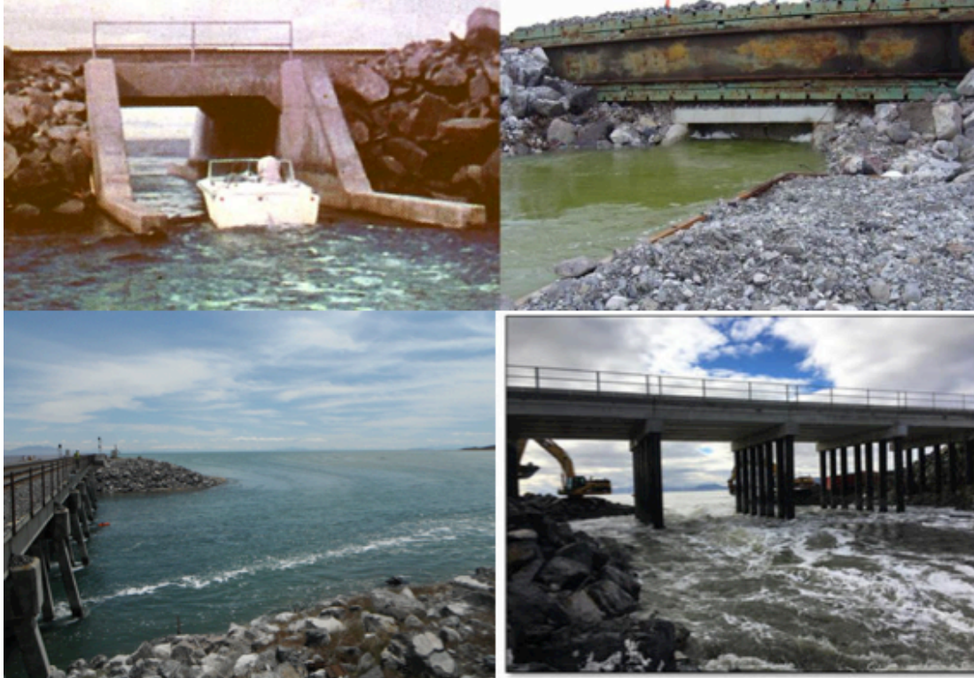
Figure 2.1. The original 15 ft wide culverts of the causeway that have been closed in December 2013 (top left and right). The breach built in 1984 (bottom left), and the breach created in 2016 (bottom right) are currently the connections between the northern and southern parts of GSL. The flow through the breaches will depend on the difference in densities and water surface elevations (WSE) between the two sides, and on the structure of the bridge. [pictures reproduced from https://usgs.gov/news and https://www.up.com/aboutup/community/inside_track/causeway-6-14-2016 ]
