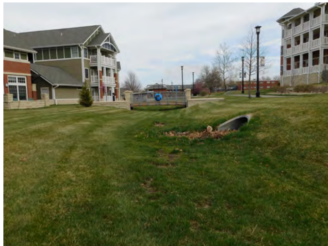
Figure 1.7. Depressed drainage area in Central Jardine.
