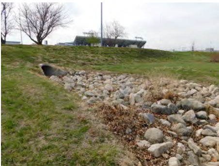
Figure 4.15. Rock swales that take on drainage from the East Stadium parking lot.
