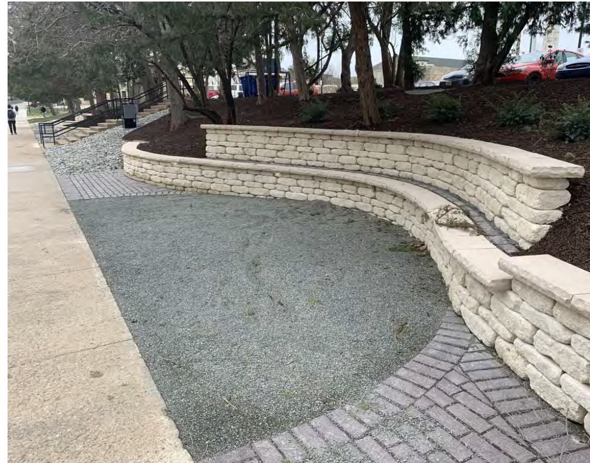
Figure 8.3. Permeable pavement at Kansas State University.
