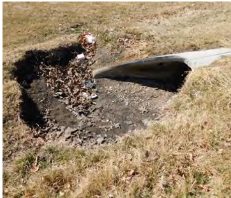
Figure 4.22 (top) and 4.23 (bottom). North Jardine Parking Lot Stormwater Outlets.
