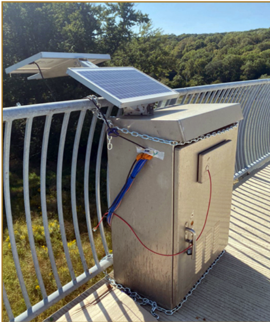
Secured cabinet at bridge deck containing DAQ.
