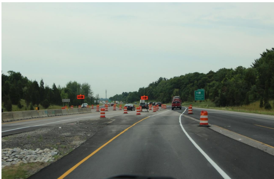
(c) Location C – right lane (mile post 173)
