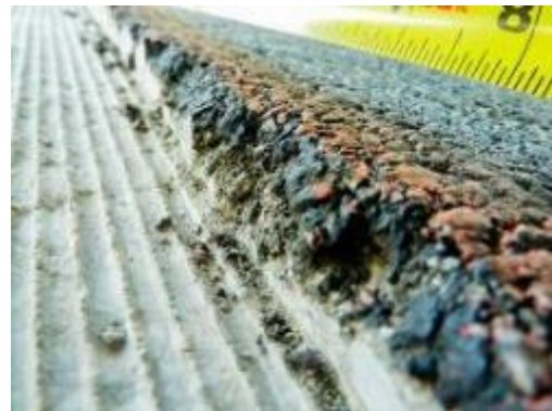
(b) Edge raveling/crumbling
