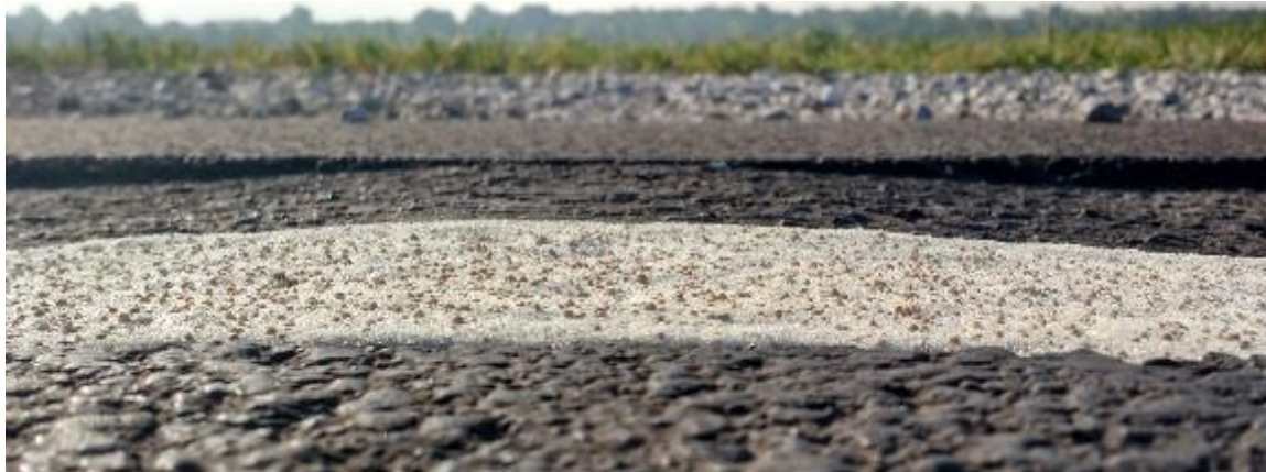
Figure 13. Close-up view of thermoplastic marking on sinusoidal rumble strips
