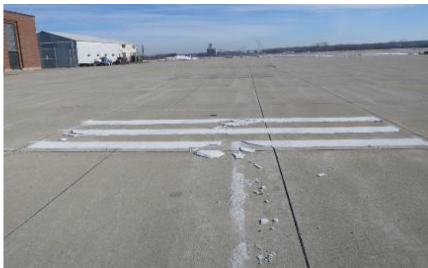
Figure 28. Cracked thermoplastic rumble strip after winter operations
