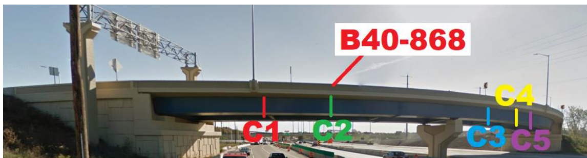
Figure 146 B40-868 Crack Locations
