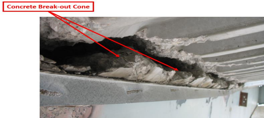
Figure 1 Neuman (2009) [3] concrete break-out failure geometry after second full-scale twin-tub-girder experiment performed
