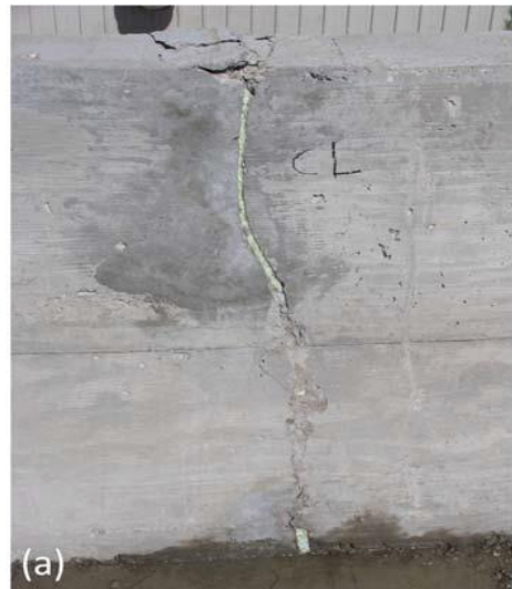
Figure 67 Parapet contact at the mid-span from Neuman (2009) [3]
