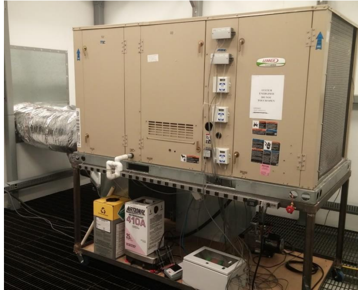
Figure 3: Lennox Rooftop Unit with 2-Stage Operation used for VRC Assessment
