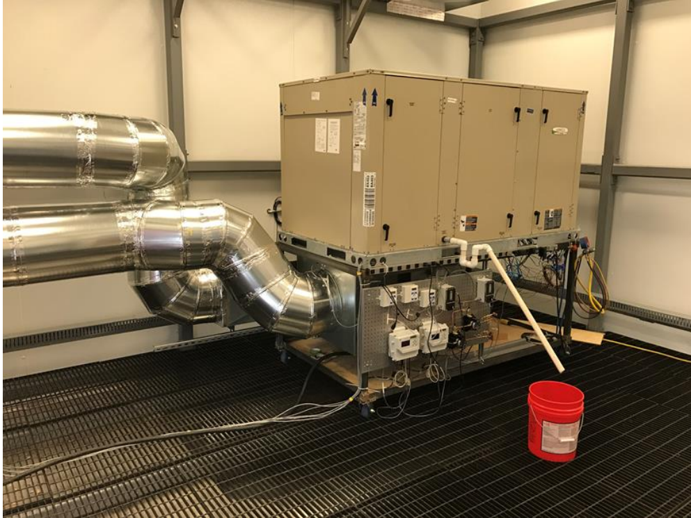
Figure 10: Lennox Rooftop Unit with Variable Speed Operation used for Charge Optimization.
