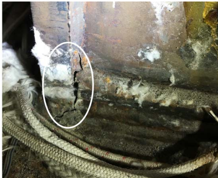
Figure 6.27 SC-W-H: Weld fracture at detail A (observed after 2\Delta_y heated cycles)
