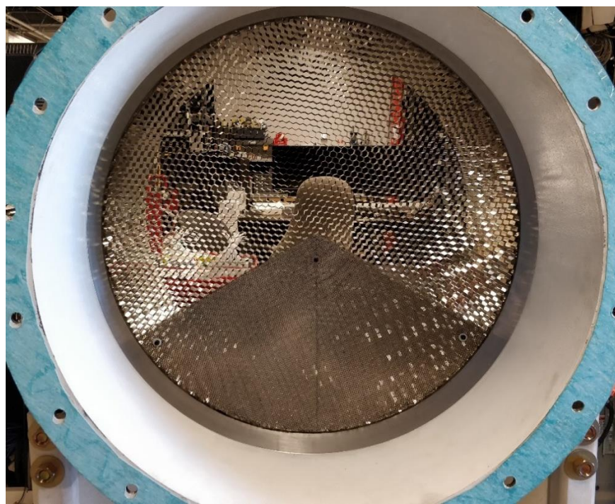
Figure 3-6. Photograph of Final Screen Candidate Installed in Traverse
