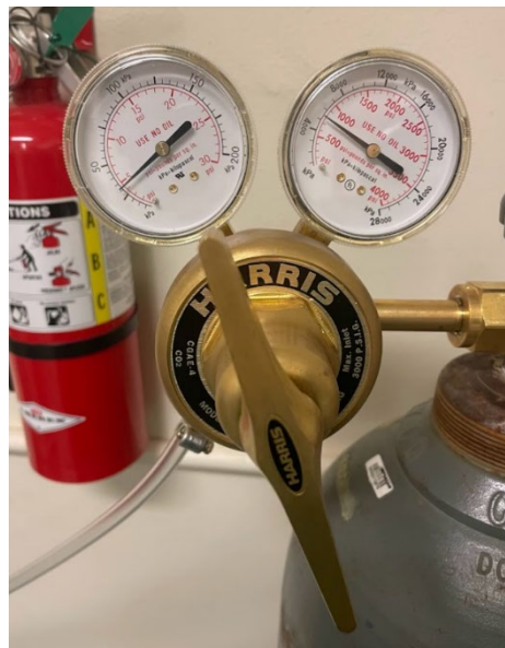
Figure 7. Pressure regulator shown with appropriate input and output pressures. The handle shown in this photo is for changing the output regulation. DO NOT rotate this handle, the control system established for this chamber is for an output pressure of 5 psi only.
