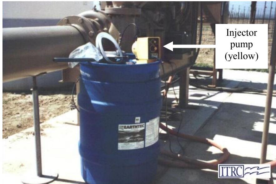
Figure 5. A small injector pump is all that is needed to add some specialty products to drip systems to minimize plugging.
