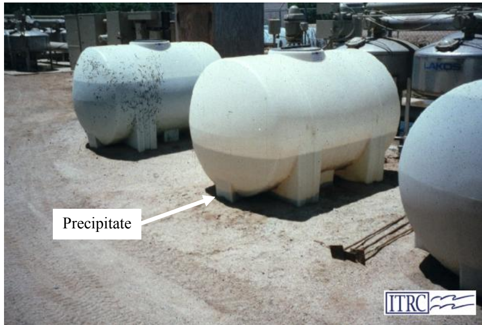
Figure 3. Chemical tanks with precipitate in the bottom. This will plug the injector pumps if no filter is installed between the tanks and the injectors.
