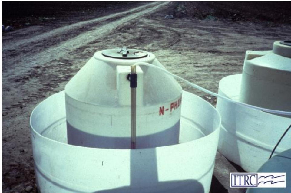
Figure 2. Chemical tanks placed inside larger containment tanks.
