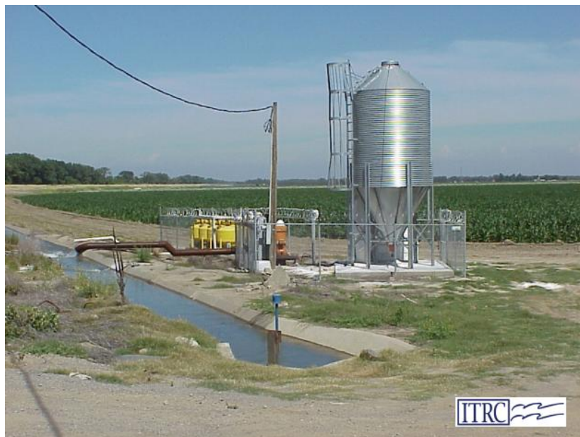
Figure 18. Large silo of gypsum powder with gypsum injection machine behind it.
