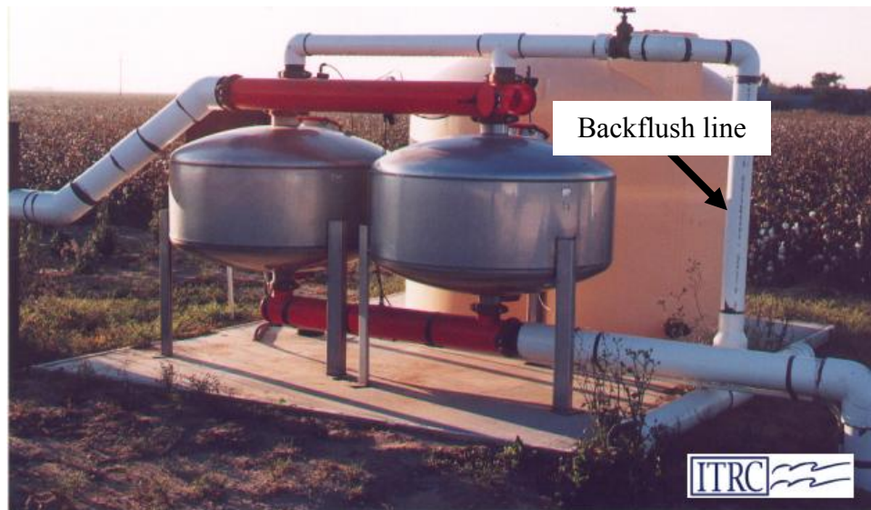
Figure 20. When filters are backflushed, injected chemicals can be lost unless the chemical injection is temporarily suspended.
