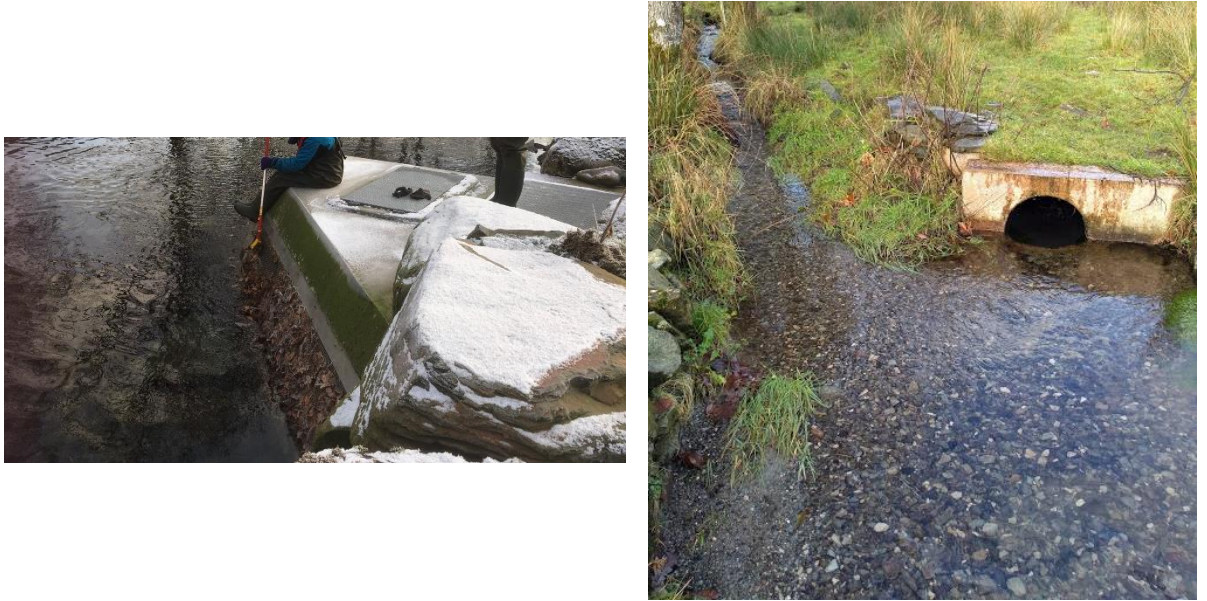
Figure 3.5 Photographs of the off-take structure (left) on the Great Langdale Beck and the discharge of the pipeline into a field drain which discharges into Elterwater inner basin (right).
