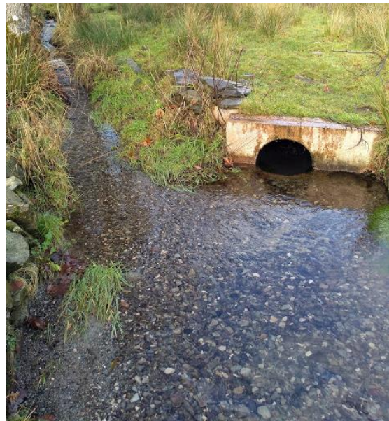
Figure S 4.7.2-1 Photographs of the off-take structure on the Great Langdale Beck and the discharge of the pipeline into a field drain which discharges into Elterwater-IB
