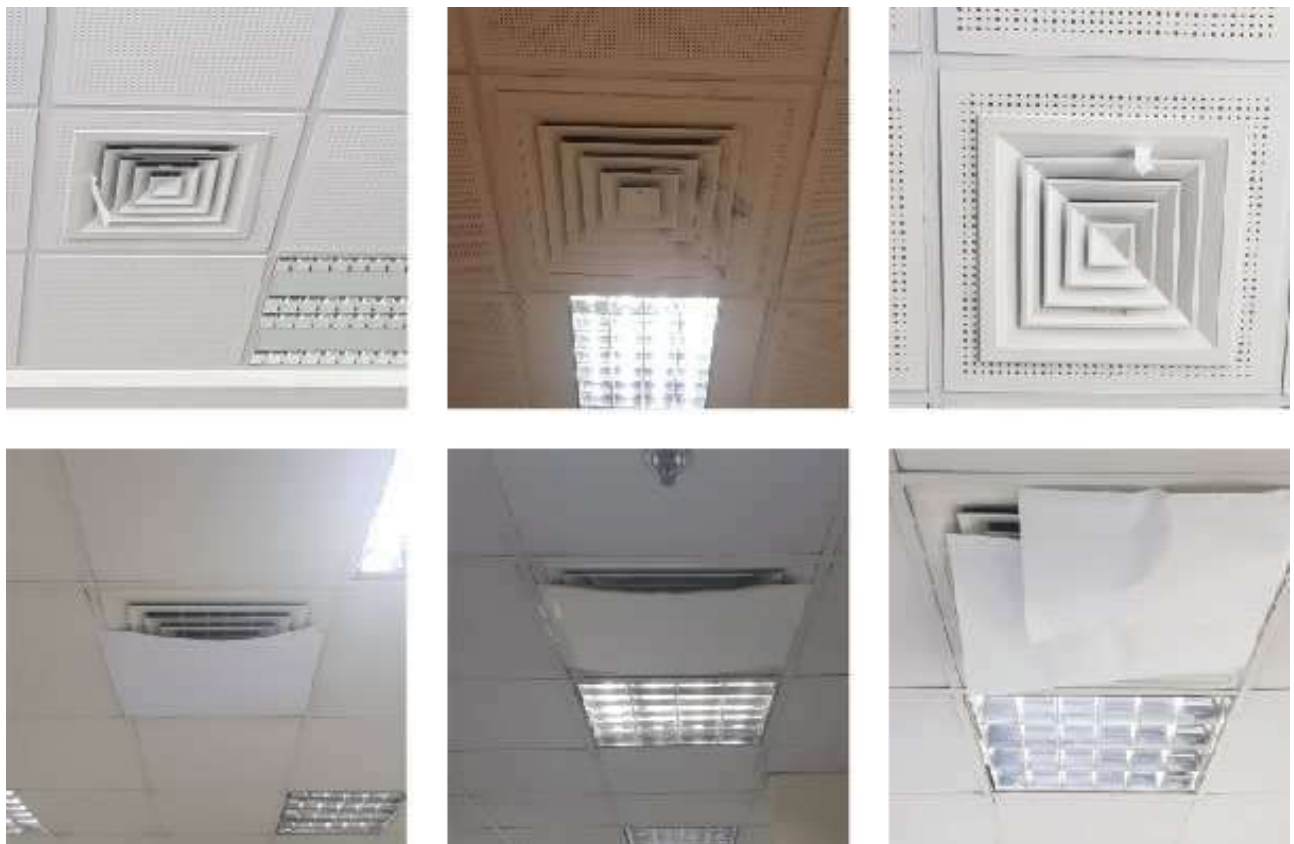
Figure 9, Images of observed occupant alterations to building air cooling distribution systems
