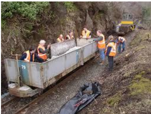
Volunteers clearing the lines in September 2017 following a period of unsettled weather and a land slip.
