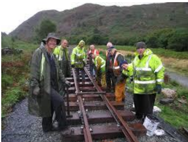
A group of volunteers at the FFR, working on repairing a section of track which was damaged in the summer of 2017.
