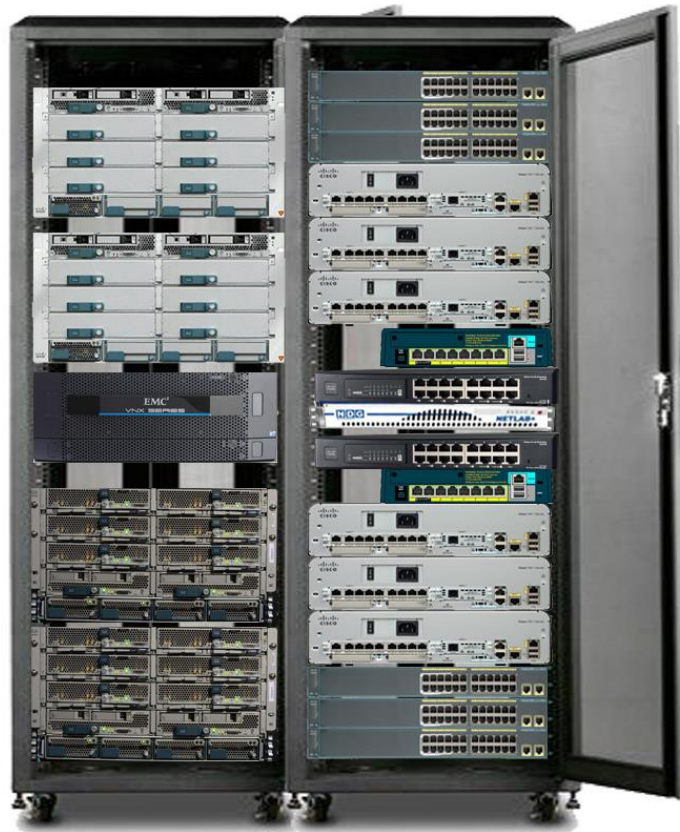
Figure 2. Initial prototype design of the VCASTLE rack mounted system.
